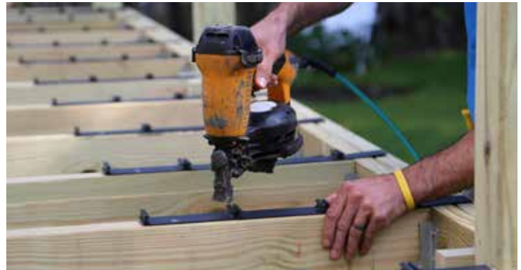
Position the end of each clip strip at chalk line and nail strips to each joist with side tabs tight against the same side of the joist.
