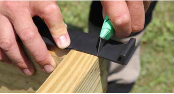
Score and trim each clip strip flush with the outer edge of the rim joist to facilitate Starter board installation.
