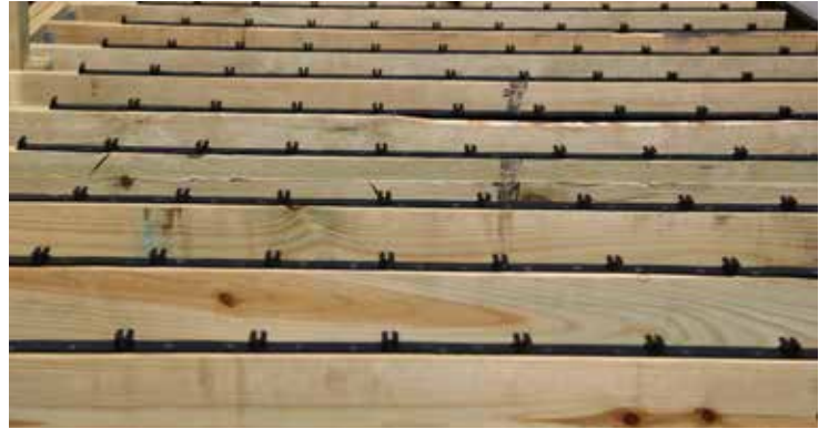
Strips may be installed on joists all at once prior to installing decking or one row at a time for elevated decks.
