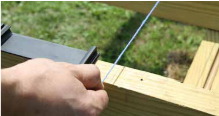
Snap a chalk line across the deck joists at a mark measured 21 5/8" (549 mm) (for 1" board overhang) from the outer edge or rim joist.
