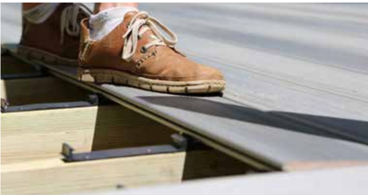
Position boards along each row of clips and step down or use a mallet on the board at each joist location to secure it into place.
