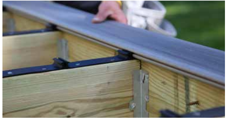
Slide starter board tightly into first set of clips and secure with composite deck screws along the outer edge of board.
